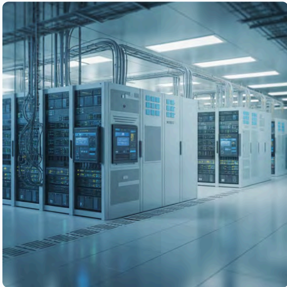
Security integration of physical systems with IT networks
